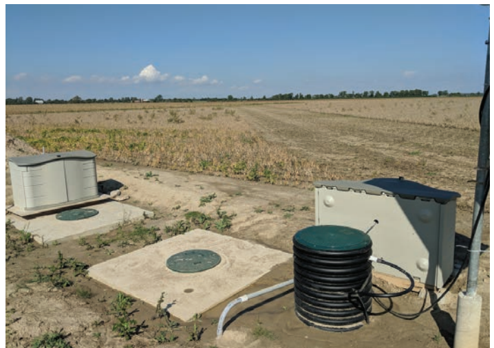
Colin Little - Agricultural Program Coordinator and Austin Pratt - Water Quality Specialist, oversee the phosphorus reduction initiatives of the LTVCA. The TRPRC phosphorus filter tank pilot project site is located southwest of Chatham near the Thames River.
