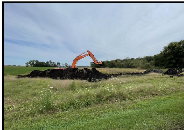
Excavation begins on a 7-acre parcel of poorly draining muck land near Highgate.
