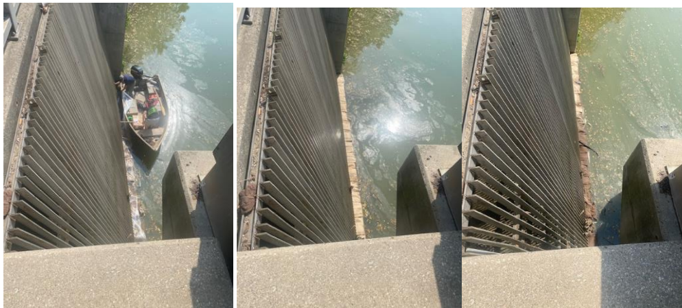
6 th St. Dam - Masen Kankula and Randy Kirby placing Storm Bags along the Dam grate
