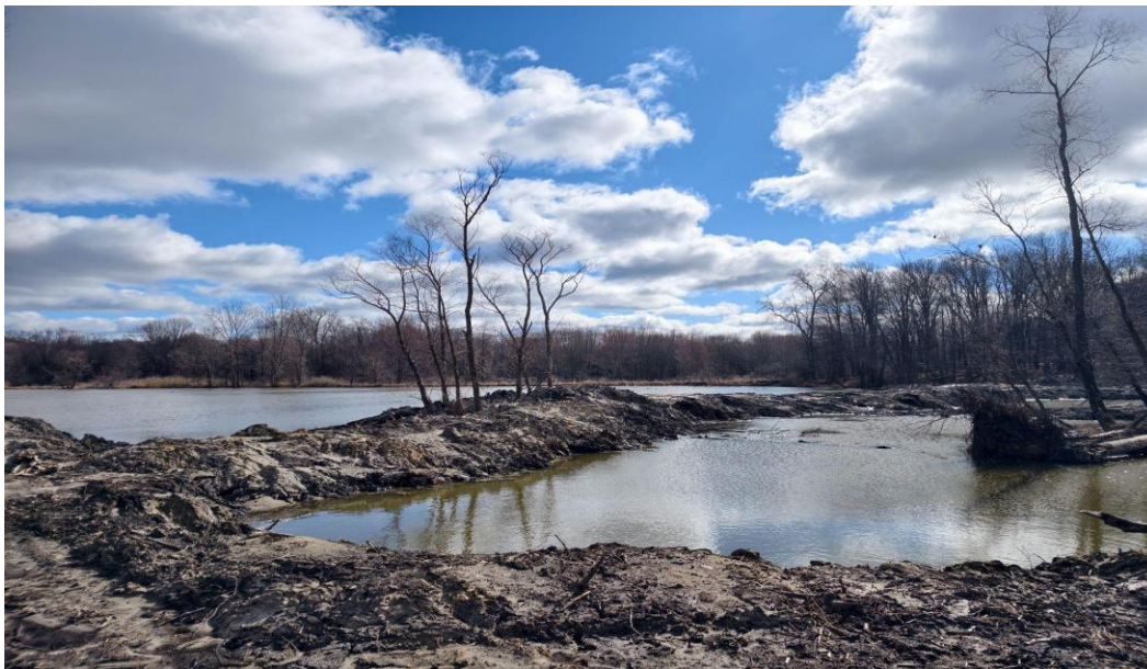
ALUS Staff inspecting a recently completed wetland project to determine eligibility for the program.
