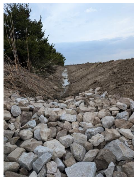
Erosion control project in Port Alma. Shown here includes grassed waterway ending in rock chute
