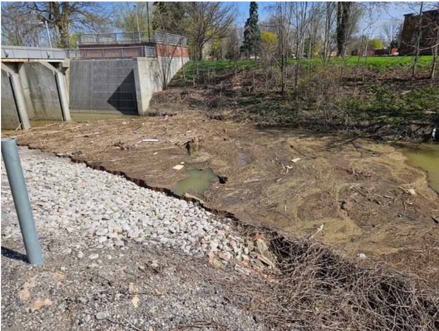
Debris at 6 th Street Dam.
